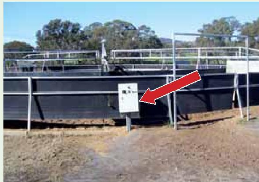
Horse walker controls are located in close proximity to gate and fitted with an emergency stop button.
