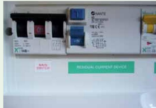
Residual Current Device (safety switches) hard wired into all electrical switch boards.
